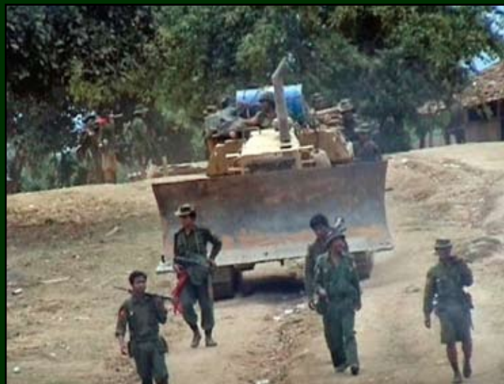
Bulldozer being used to clear new roads in Nyaunglebin and Papun Districts. April 07.
